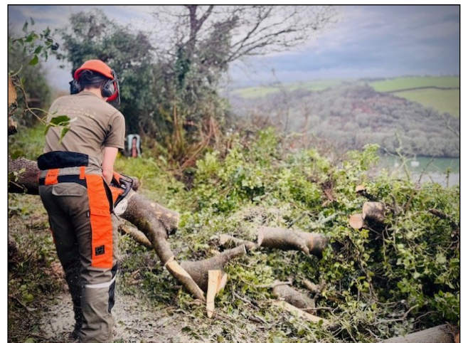
Hard at work clearing fallen trees on the Upper Downs, high above our beautiful River Fowey.
